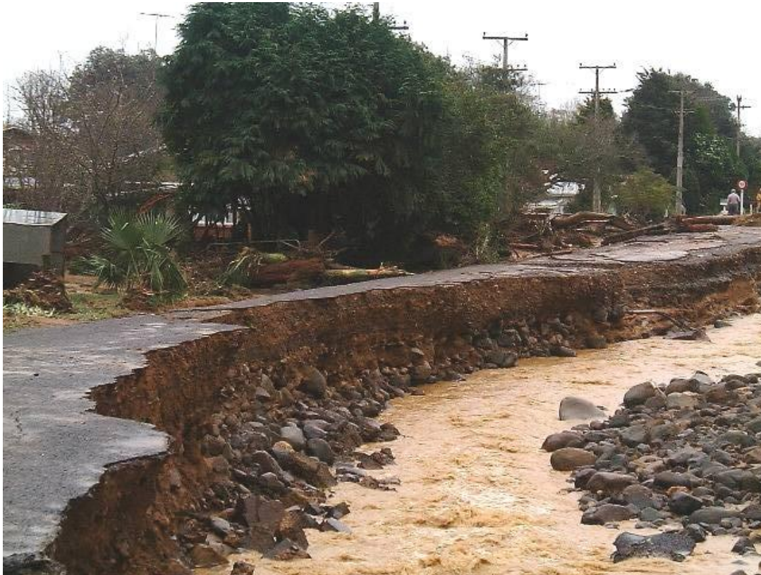
Photo 1 Te Puru Creek Rd erosion following the 2002 flood. View looking downstream.
